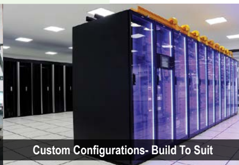
Industry Compliant Production Capabilities
