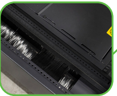
Brush cable managers in floor of cabinet
